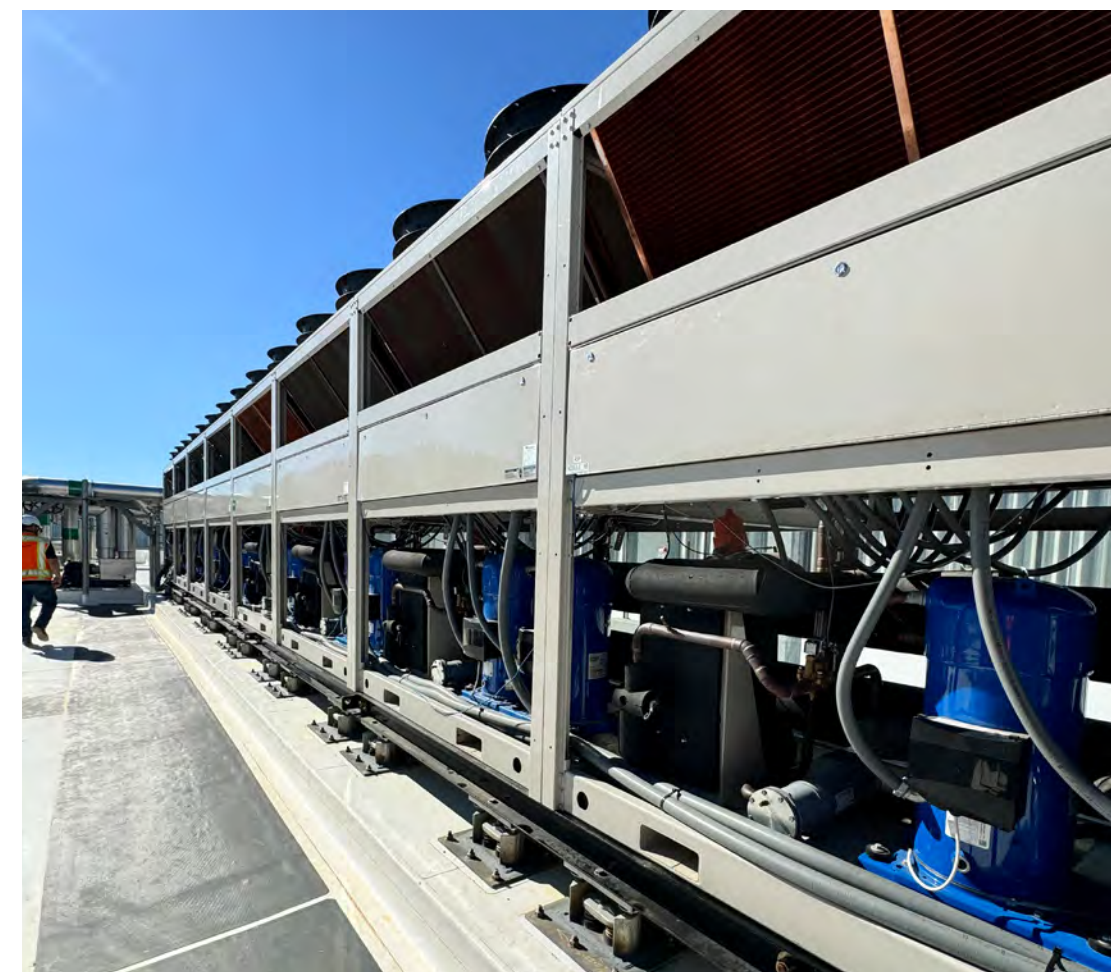
Multiple 4-pipe air-to-water heat pumps stacked together for 480 tons of cooling and 240 tons of heating.
