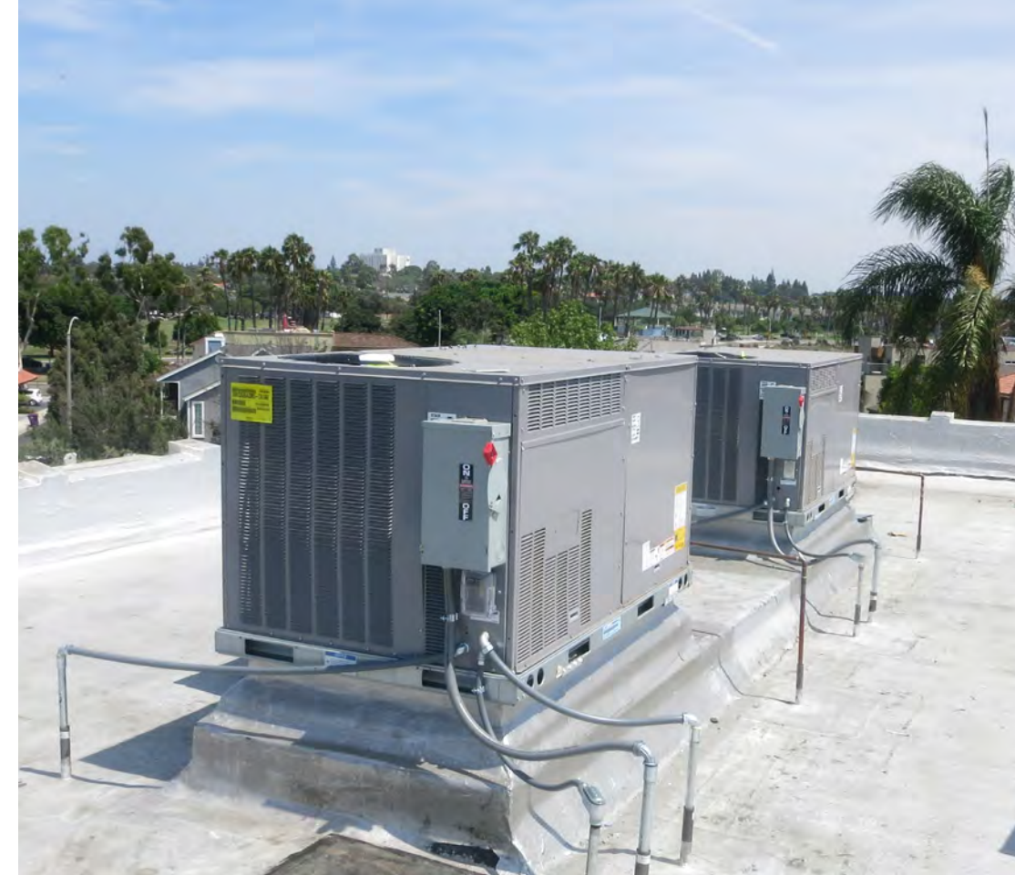
5 ton rooftop heat pump.
